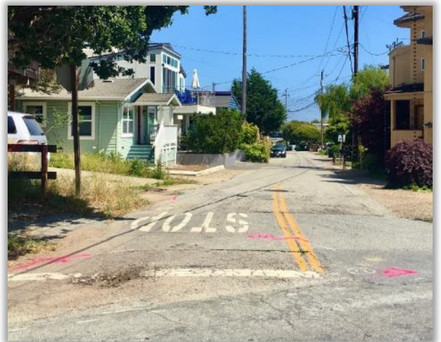
Hillcrest Drive at Mar Vista Drive is marked for Measure D resurfacing this summer.
