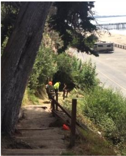
Using materials purchased with SIA funds, State Park staff replaced railings on a section of the Beachgate Trail.
