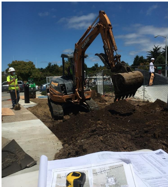
A smaller excavator still requires skill and steady steering to clear space for the new restroom adjacent to the recently installed skatepark.
