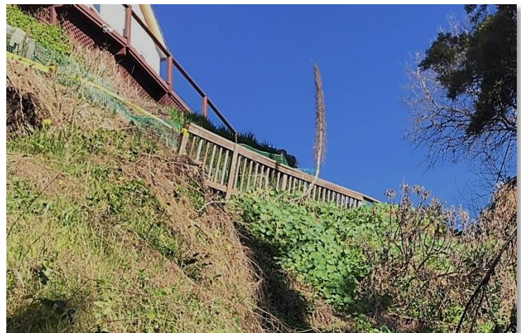
View of the damaged Beachgate Trail railing from below.
