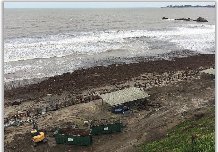
Storm damage clean up at Seacliff State Beach.
