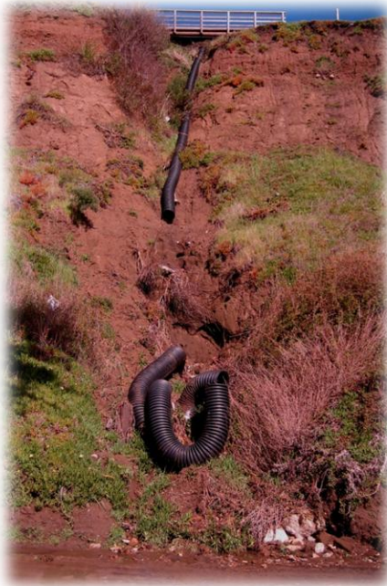
Storm Drain Damage in February 2010 The cliff is still relatively intact with the tube resting on top of the slide.
