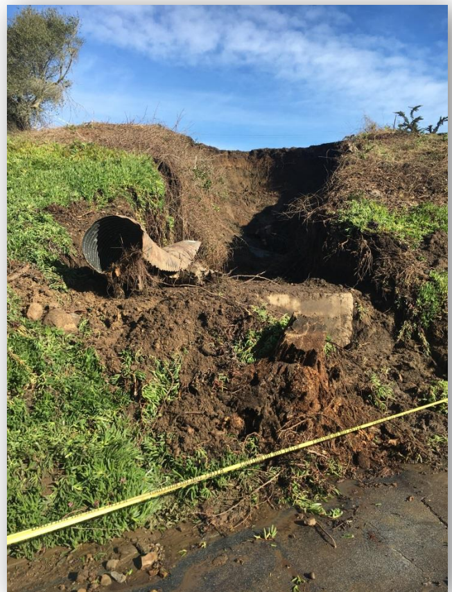
These are the remains of the storm drain at the entrance to Seacliff State Beach that failed during a winter storm in January, 2017. Repairs and replacement of the drain pipe was completed immediately because the location of the damage was within six feet of the main Seacliff sewer line. Other Seacliff storm damaged sites are still awaiting repair.
