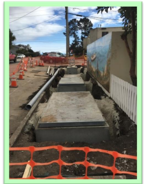
Construction of utility boxes required great care next to the Seacliff mural.
