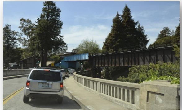
Pedestrian sidewalks on Aptos Creek Bridge are too narrow and close to vehicle traffic.
